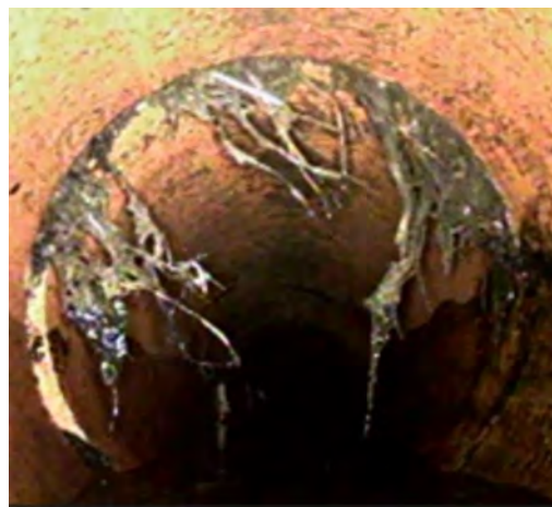
View of Root Intrusion by the Robotic Sewer Televising Camera - The EnviroSight ROVVER X sewer televising camera captured this image of root intrusion within a Village sanitary sewer pipe. The growth of roots into the sewer pipe can cause blockages or mainline breaks. Routine sewer rodding maintenance clears sewer pipes of ingrown roots to maintain patency.
