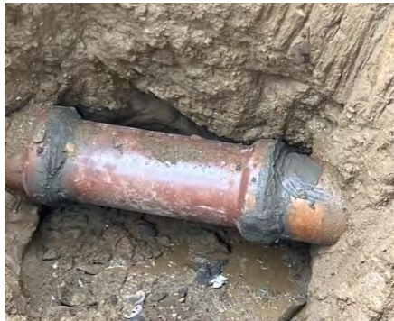
Sanitary Sewer Joint Repair on Main Street - Joint leakage in the sanitary sewer pipe resulted in the development of a sinkhole in the pavement. Excavation was completed to re-seal the sewer joints with hydraulic cement.
