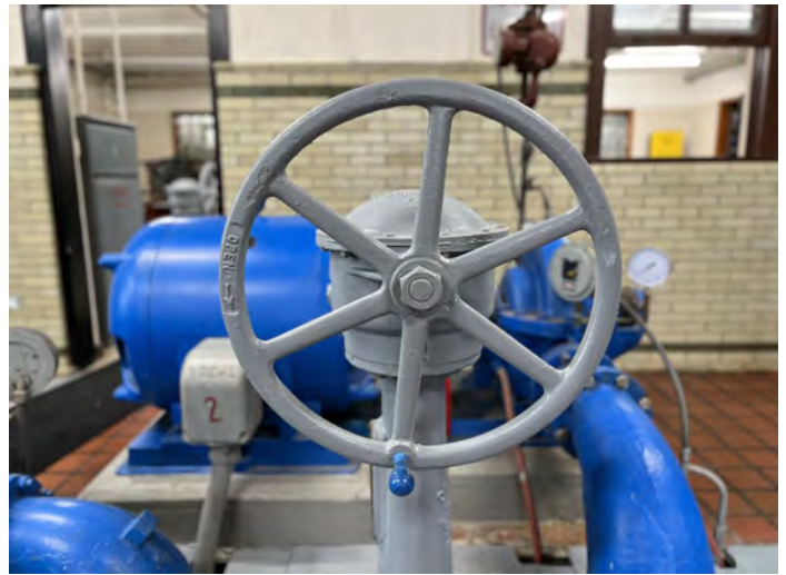
North Pumping Station Intake Valve - This North Pumping Station intake valve allows water to be pumped from the underground reservoir into the Village water distribution system.
